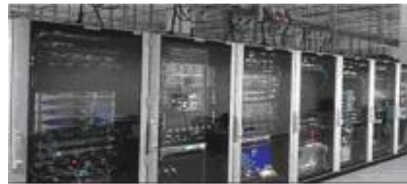
Fig. 30. The physical NIPR JRSS stack - 20 racks [31]
